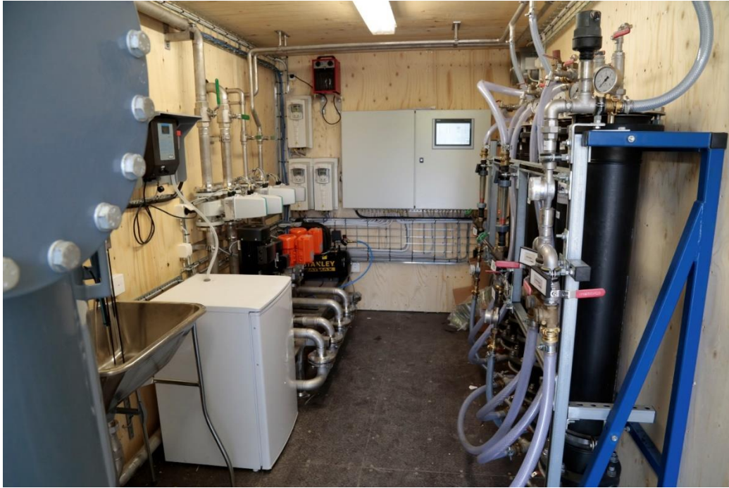
Figure 11 Picture of inside the Pre-treatment container, sandfilter (left), sampling and pumps (left), control system (mid), Cornelsen GAC-filter (right)
